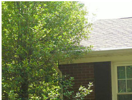
Tree in contact with the home
