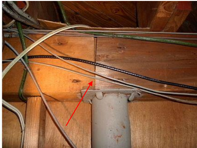
Column not completely centered beneath beam joint
