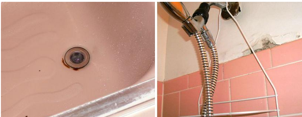
Tub drain corrosion and wall damage in bathroom
