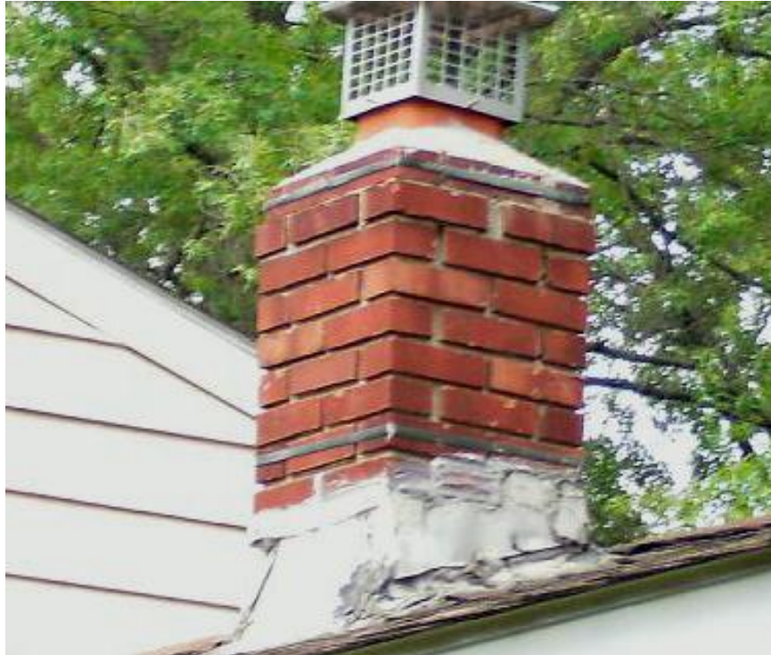
Chimney needs maintenance
