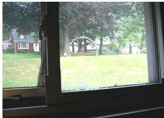
Broken glass at basement window
