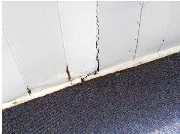
Damage to wall in enclosed rear porch caused by water intrusion
