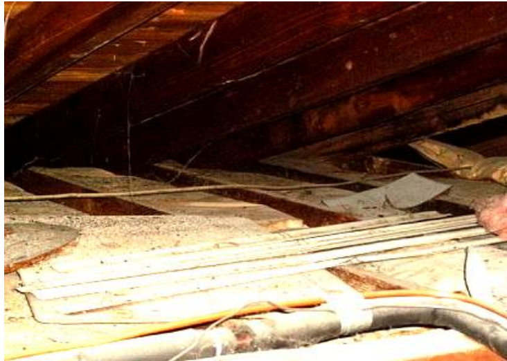
Insulation extends to the roof edge blocking ventilation, and roof sheathing boards are stained from water
