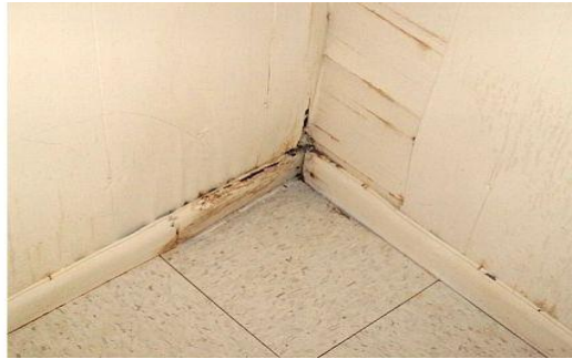
This area of basement wall tested wet
