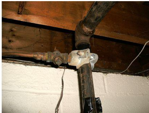
Clamp type gas pipe connector may develop leaks
