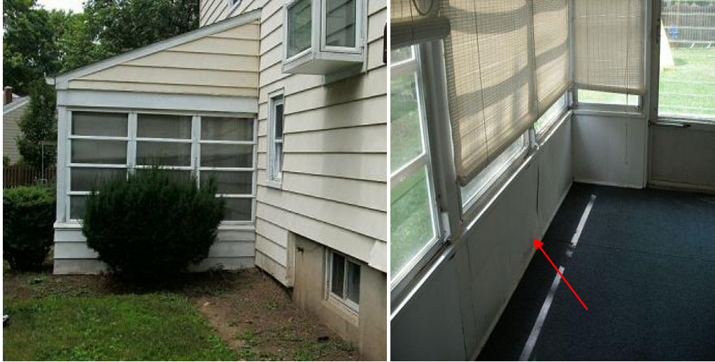
The walls for the rear attached room are damaged from water intrusion
