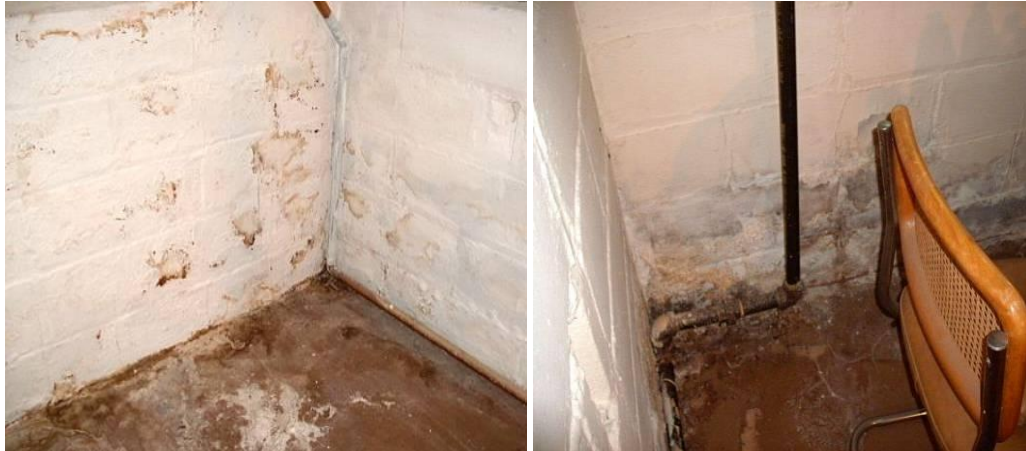
Evidence of Water Penetration of the Foundation Walls seen in Basement
