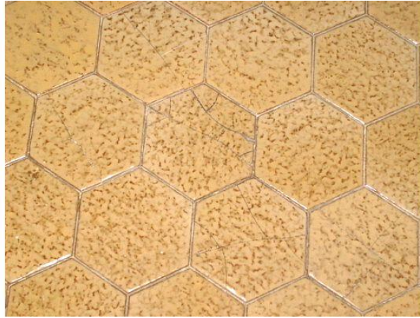
Cracked floor tile
