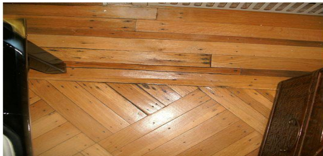
Worn Finish Flooring
