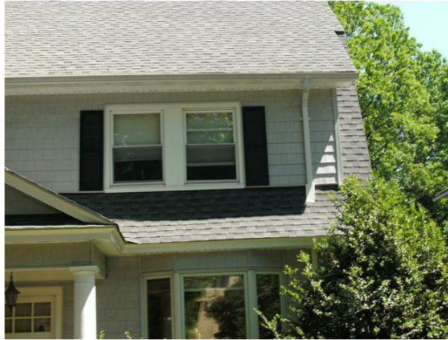
No gutters on lower section of roof
