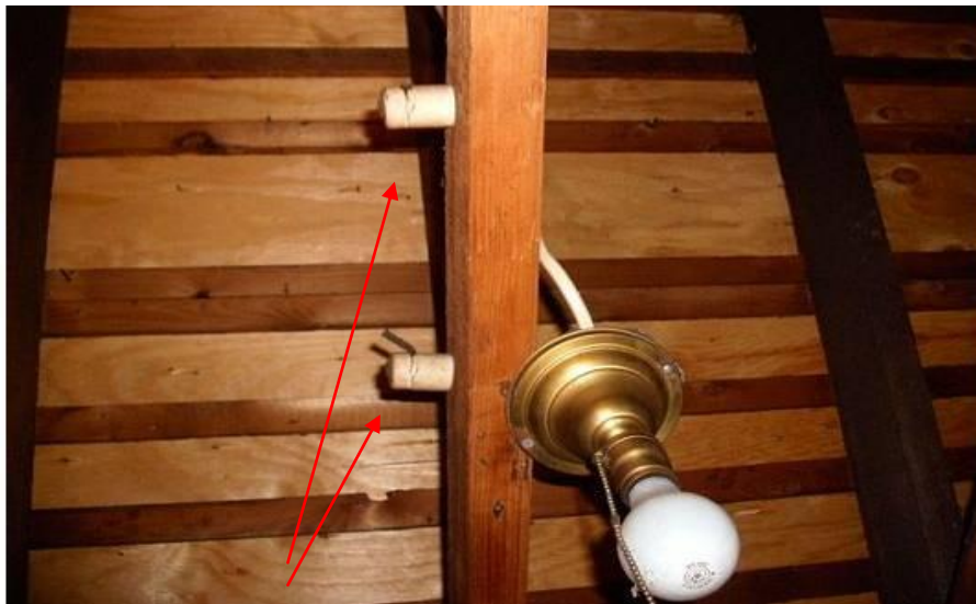
Evidence of Removed Knob-and-Tube Wiring in Attic
