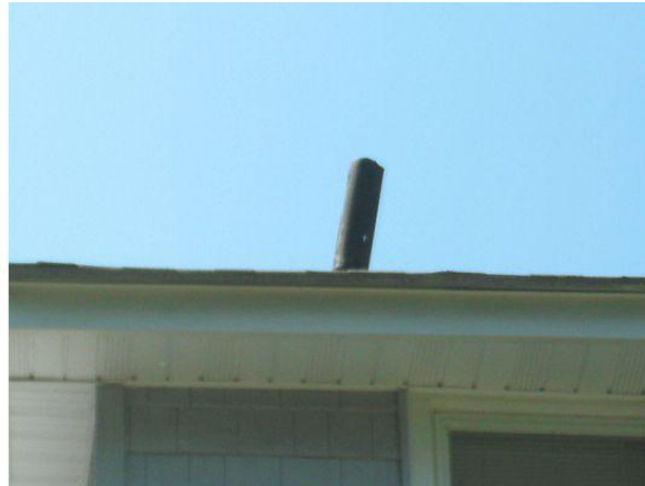
Tilted plumbing vent stack
