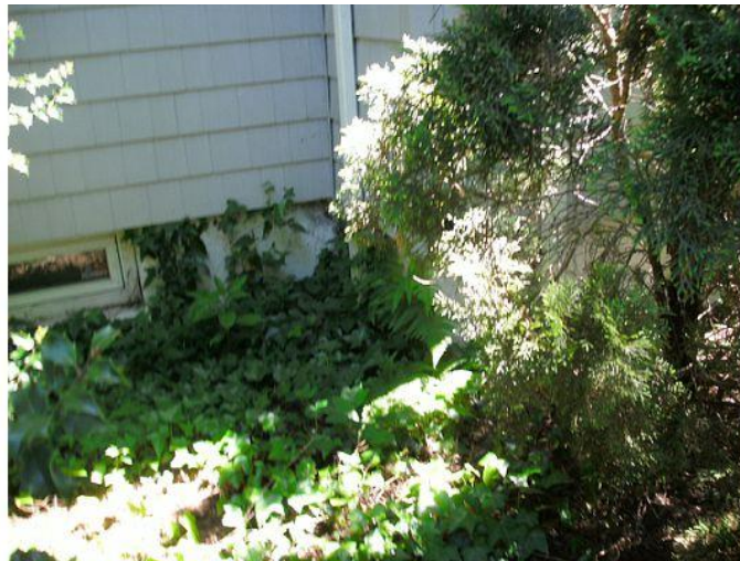
Overgrown vegetation in contact with home
