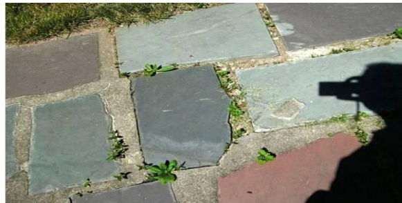
The worn patio
