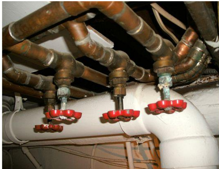
Corroded shutoff valves
