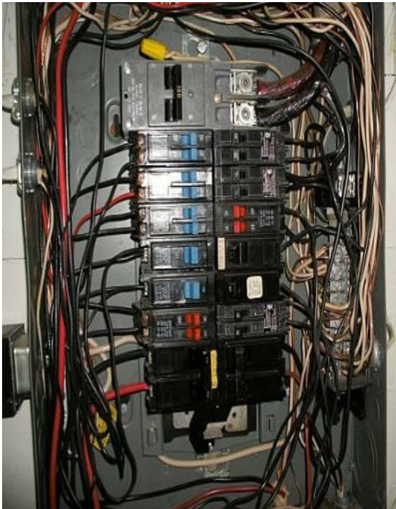
Crowded Main Electrical Panel
