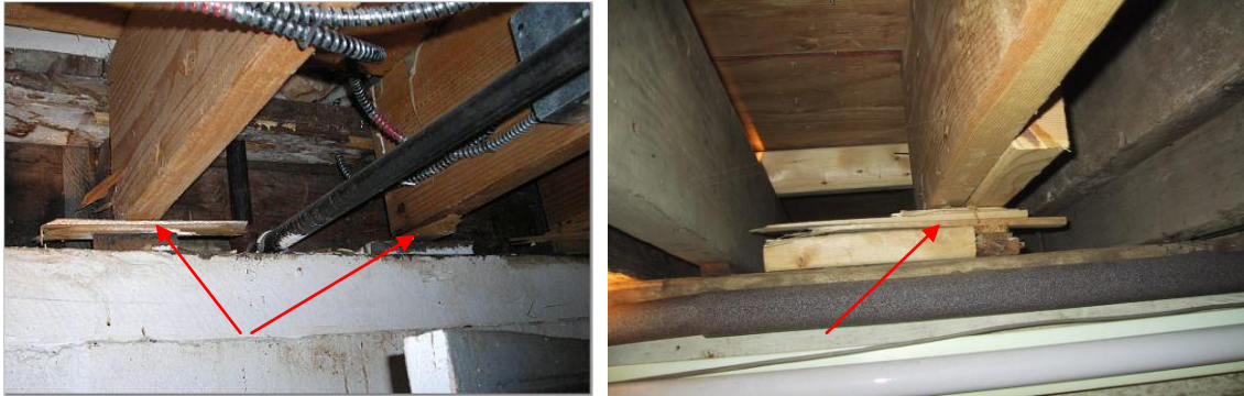
Random scraps and shims support joists in rear section of the home
