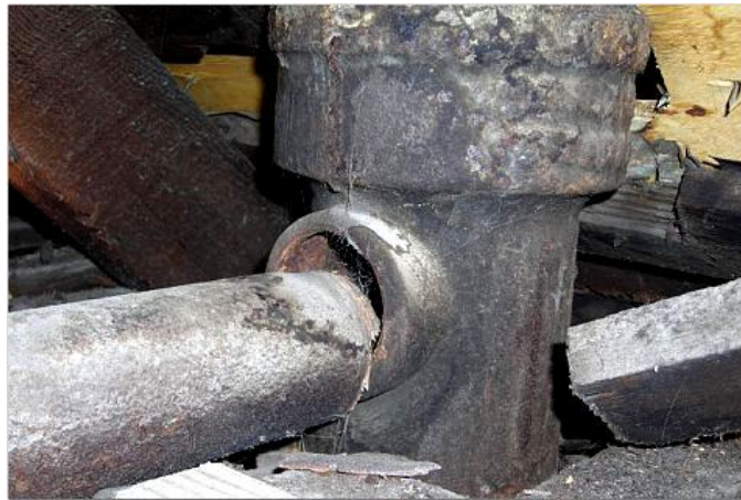
Drain Vent pipe in attic disconnected from stack
