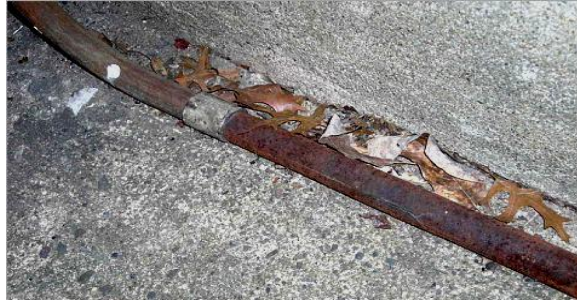
Corroded electrical conduit
