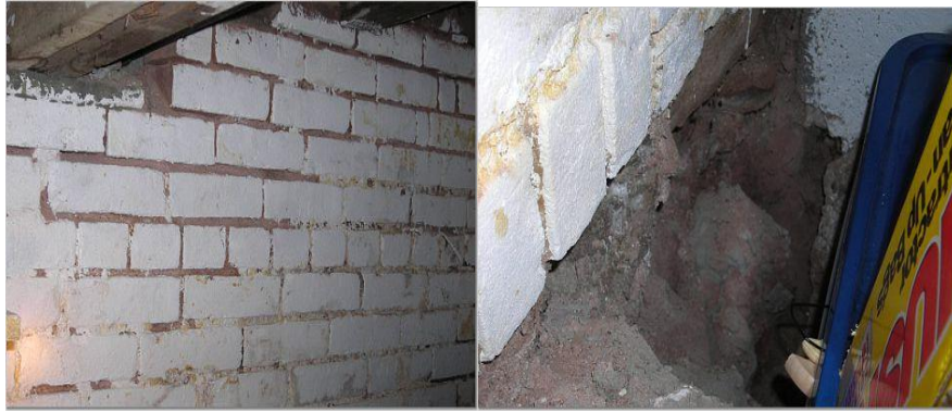
Deteriorated mortar and loose stone in foundation
