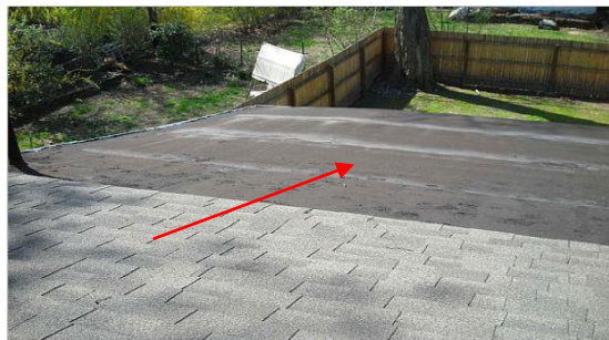
Rear low sloped roof has no protective paint
