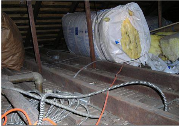
Insulation is not installed
