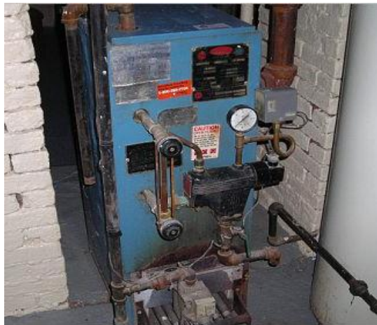
Aging heating system with corrosion and scorching
