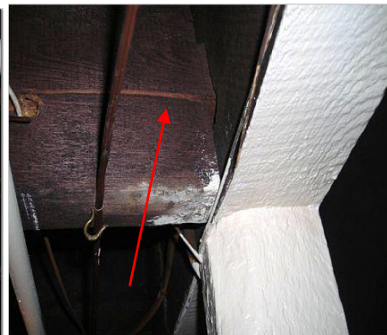
Joist cracked at tenon joint
