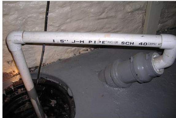
Sump pump discharging directly into plumbing drainage system
