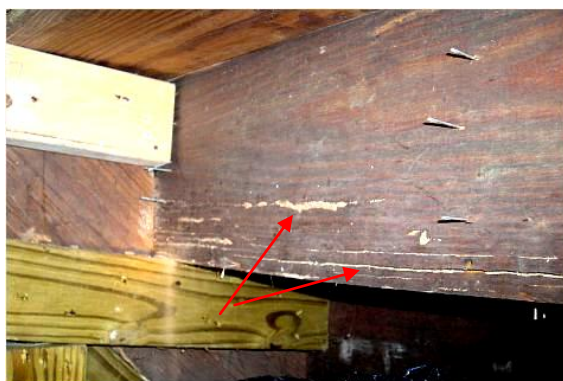
Termite mud tubes are present beneath basement stairs
