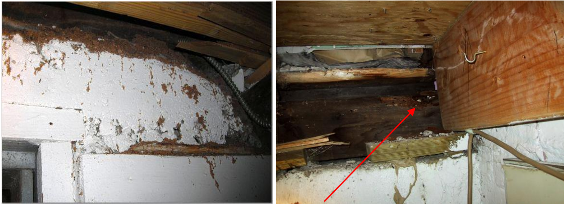
Significant carpenter ant frass, and damage to old sill plate at left rear
