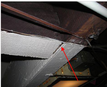
Mortise and tenon joint with gap
