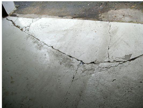
Cracked garage floor slab
