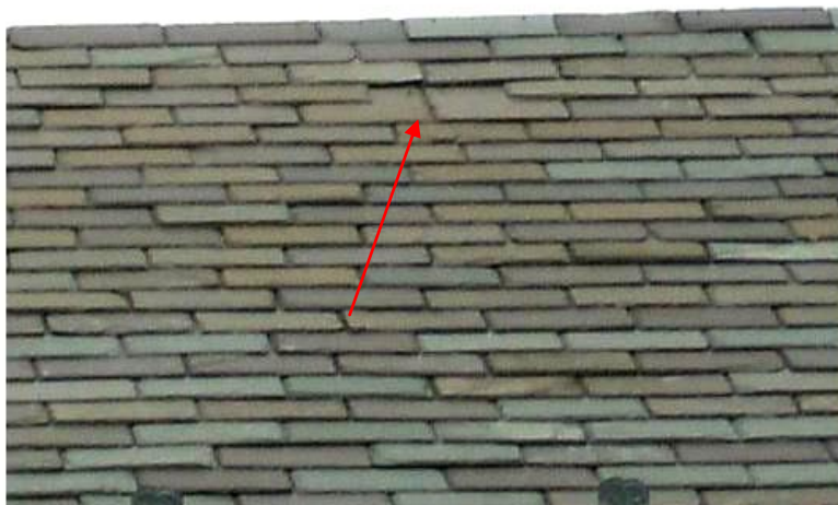
Example of Missing roofing slate
