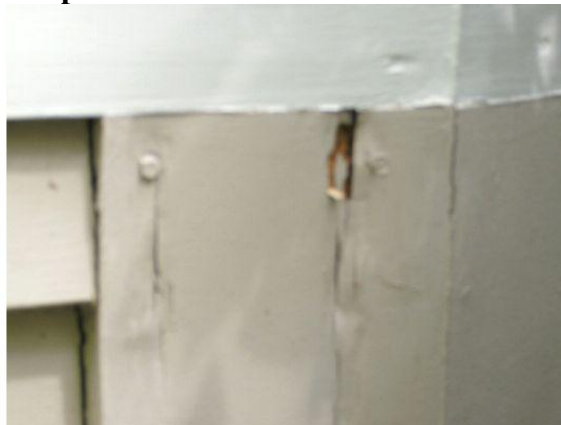
Water damaged bay window trim
