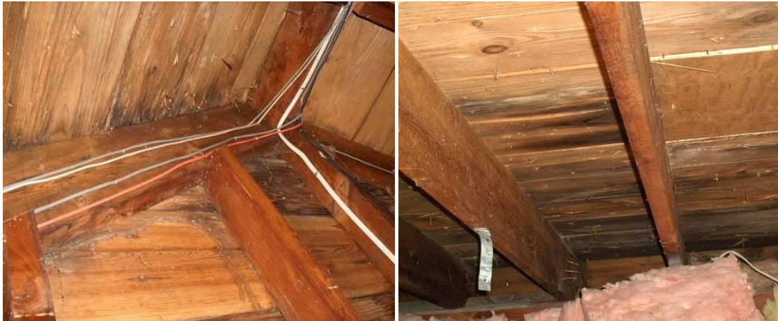
Staining on the underside of the roof / in attic suggests leakage
