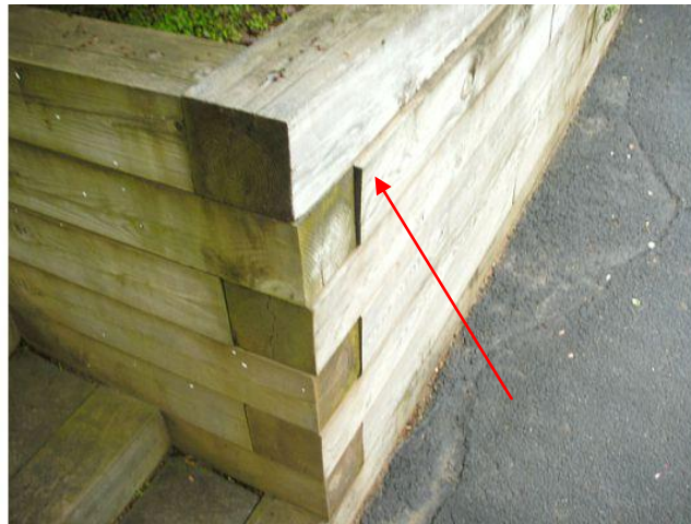
Some displacement of wood tie retaining wall
