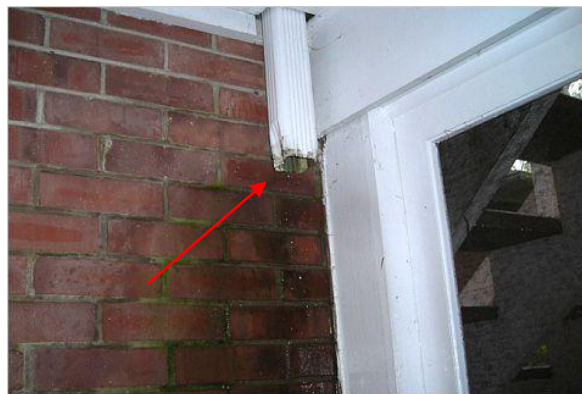
Disconnected downspout discharging into patio area
