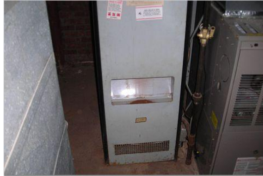
Very old heating system – note corrosion at front
