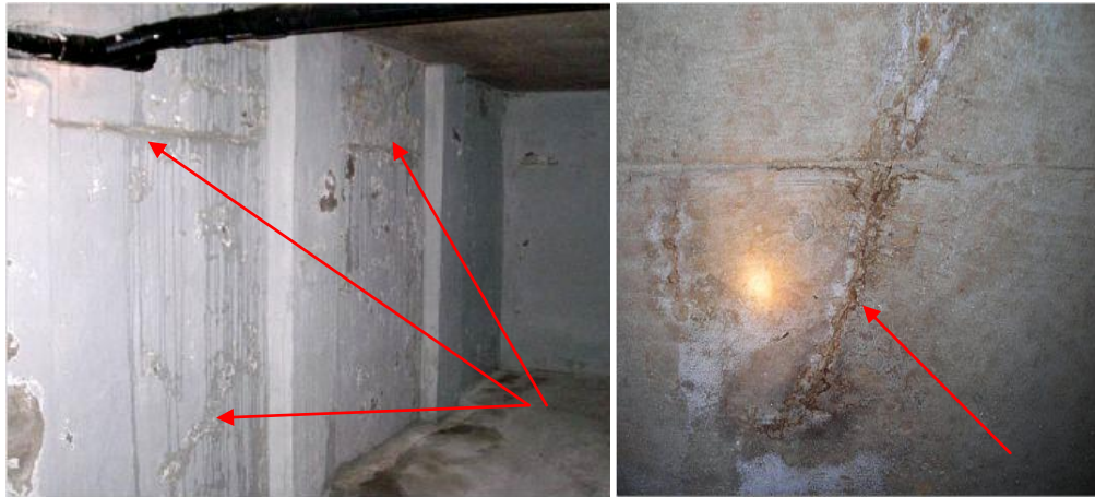
Water Entry & Damage to the Masonry Foundation at Front and also Crack and Water Entry thru Ceiling
