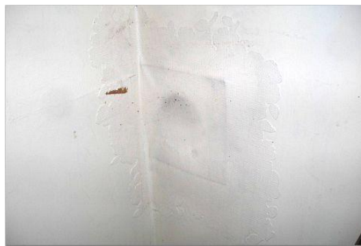
Closed over dryer vent outlet
