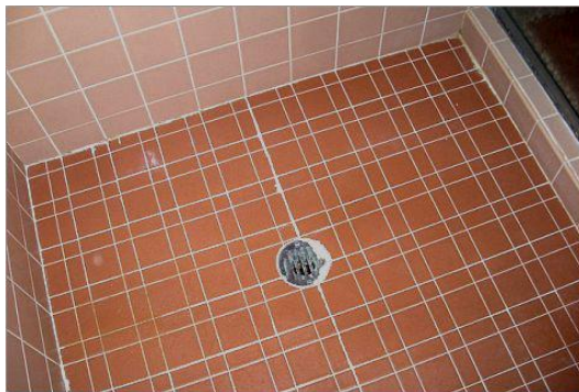
This older tile floor is likely leaking
