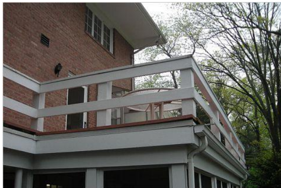
This style railing is no longer considered to be acceptable
