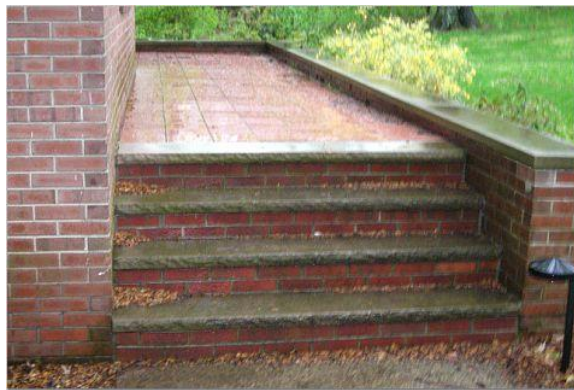
Front entry area is sloped to drain water to front, where it accumulates The area beneath this entry is a full height crawlspace
