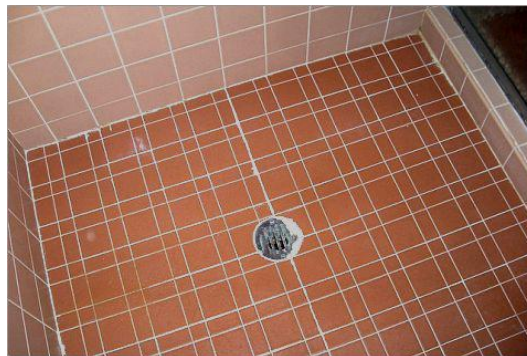
This older tile floor is likely leaking
