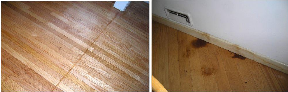
Defects in Finish Wood Flooring
