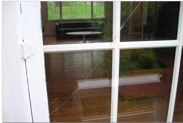
Window with cracked glass, also painted shut
