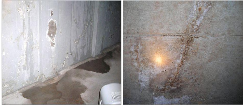
Signs of leakage through foundation wall and ceiling – front entry area is above
