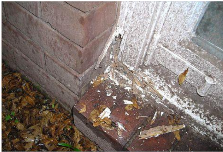
Termite damaged trim
