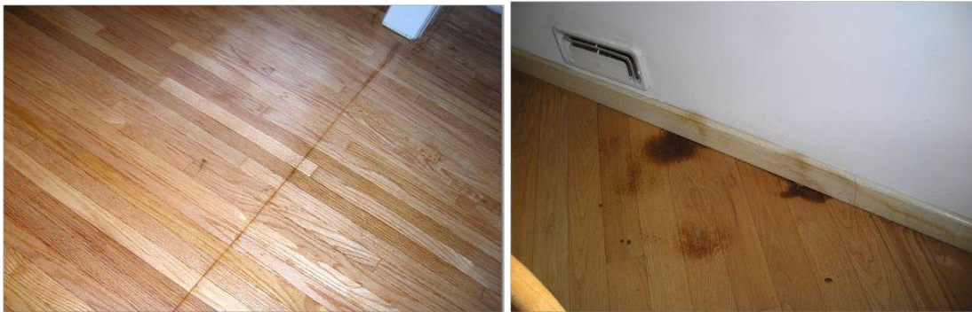
Defects in Finish Wood Flooring
