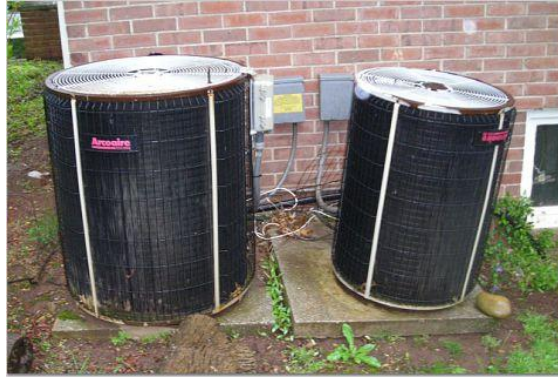
Older central AC compressor/condensing units have limited if any remaining life
