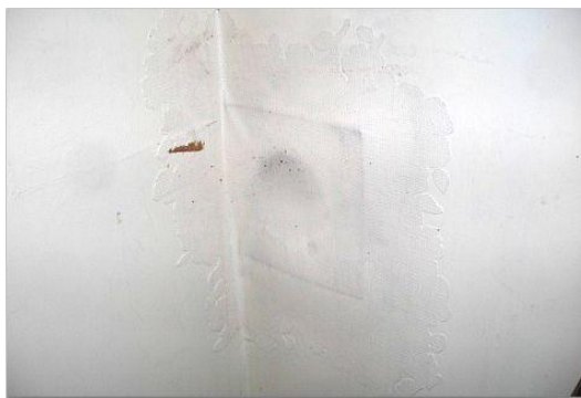
Closed over dryer vent outlet
