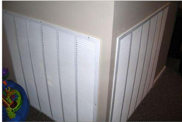
Heating system is behind fixed grills – even with grills removed, system could not be adequately serviced
