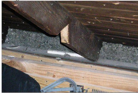
Notched rafter is weakened
