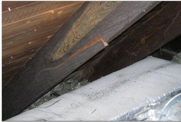
Cracked roof rafter
