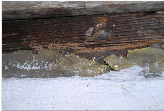
Termite damaged sill plate
