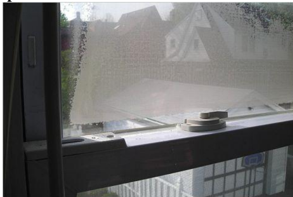
Condensation stained window
