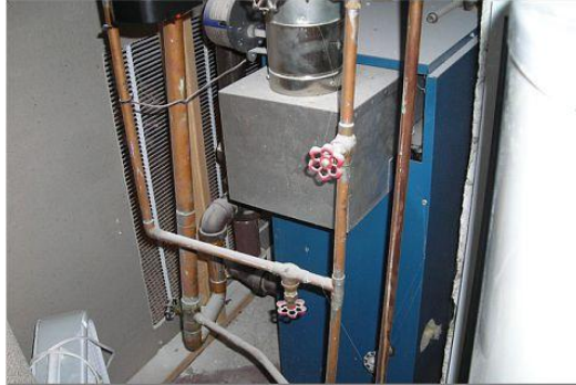
The back of the heating system – Front was not accessible or visible
