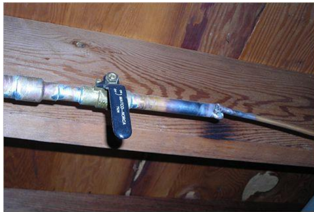
Poorly done connection
