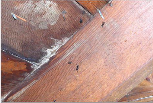
Live ant activity in stained area under roof
