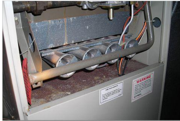
Furnace is aging and has corrosion
