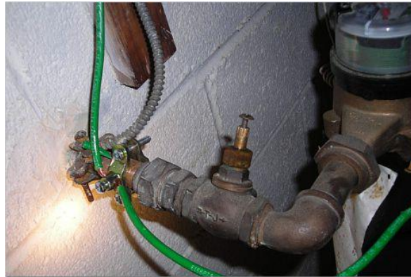
Missing main shutoff valve knob
