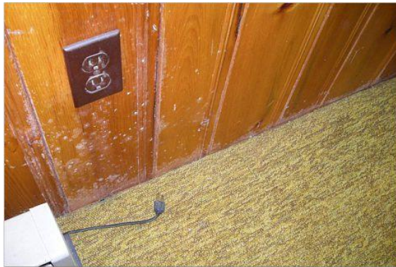
Spotting from mold growth on wood panels
