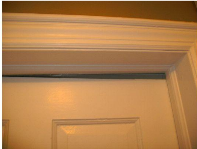
Gap at top of door
