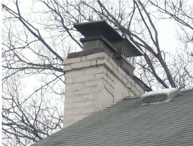
Deteriorated masonry joints at top of chimney
