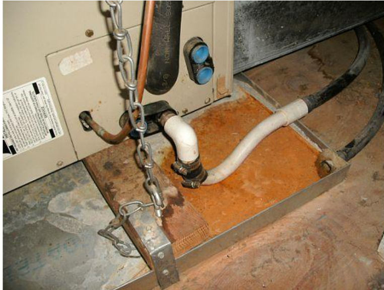
Corrosion in AC condensate drainage pan
