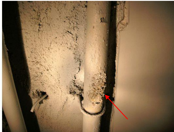
Leaking brass water pipe found in garage
