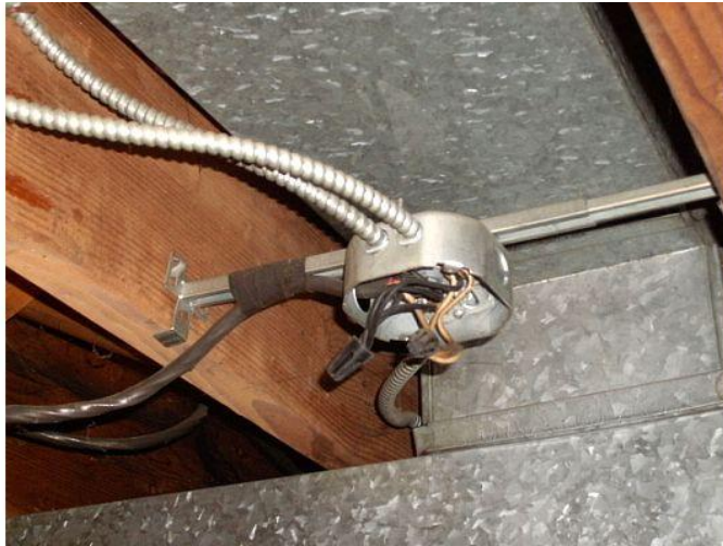
Open junction box with exposed wiring
