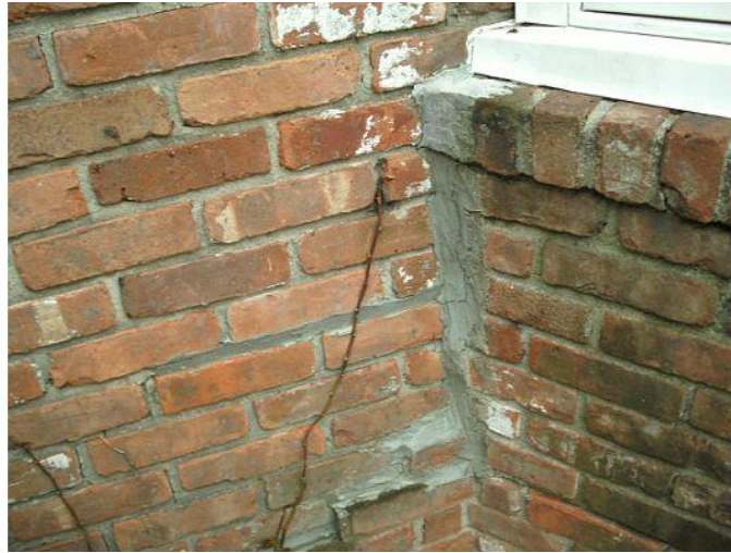
Patched cracks at the left front brick facade
