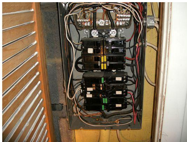
Obsolete breaker panel with no single main breaker
