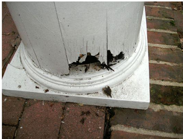
Water damage to the base of wood columns
