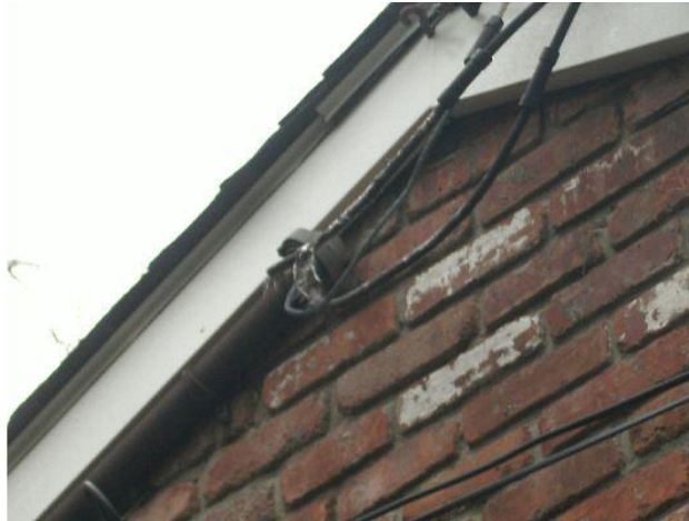
Frayed insulation on electrical service entrance cable
