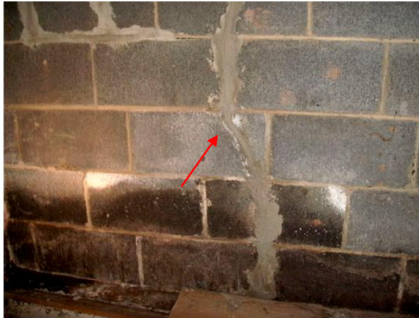
Patched cracks in foundation wall visible in crawlspace
