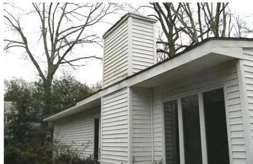
No rain gutters present on most sections of the roof
