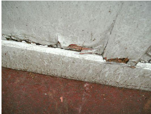
Damage to garage door
