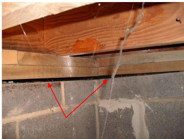
Gap between foundation and sill plate
