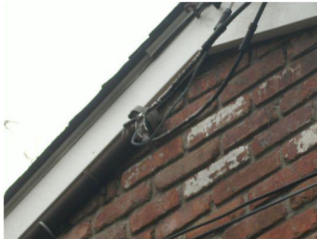
Frayed insulation on electrical service entrance cable
