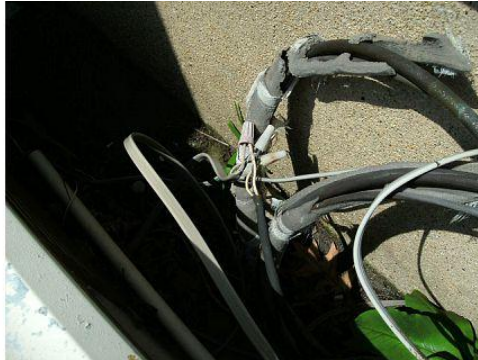
Exterior AC connections are exposed
