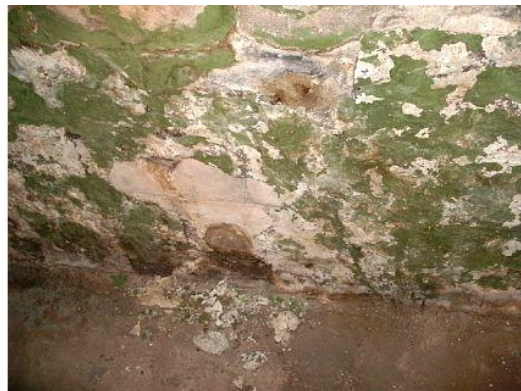
Crumbling interior foundation wall coating
