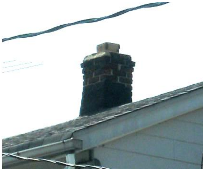
Chimney has heavily tarred and patched flashings and needs repair
