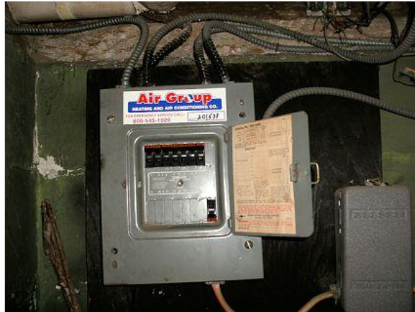
Federal Pacific breaker panel – known to be unsafe
